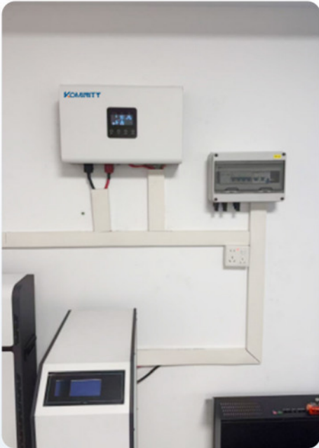
6kW Installation Case -Poland
