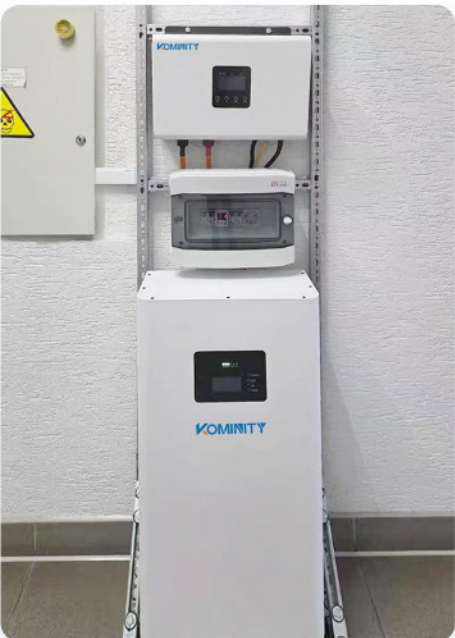
6kW Installation Case -Nigeria
