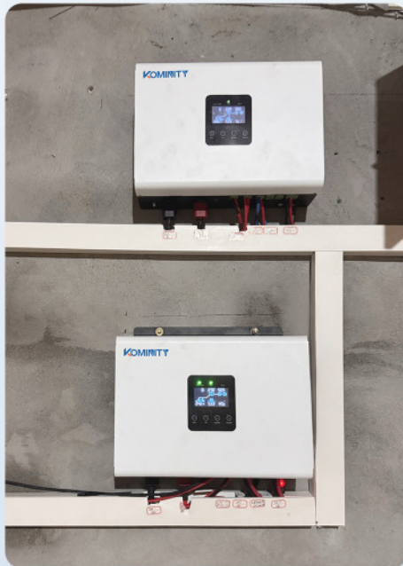
6kW Installation Case - Vietnam
