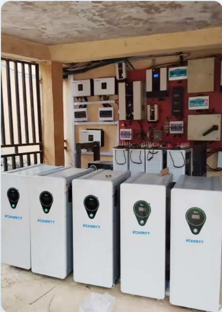
12kW Installation Case -Myanmar
